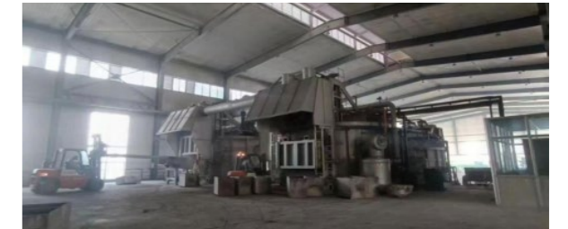
Comprehensive Utilisation Equipment of Aluminium Ash
